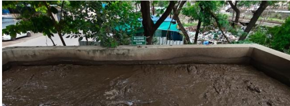
Sludge Blending tank
