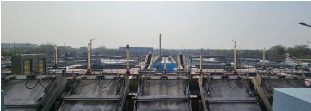
Collection, screening and grit removal
