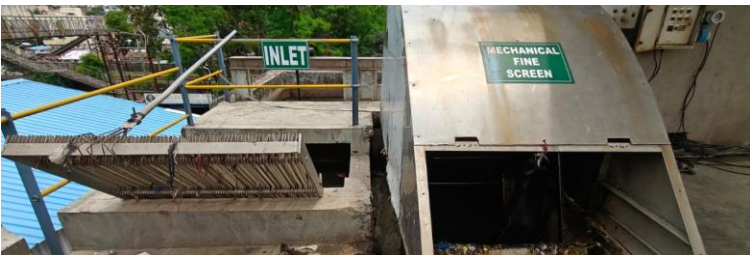
Screen and Grit chamber
