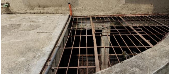
Incoming Sewer and pumping station
