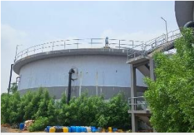
Primary treatment- Clarifloculator
