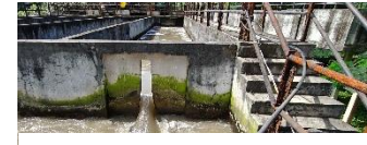
Outlet after screening
