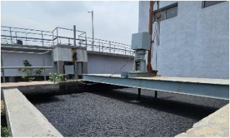
Sludge thickening tank
